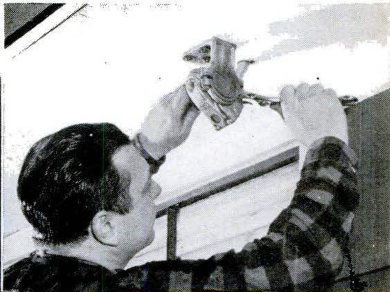
TWO BOLTS were tightened to clamp the gear case into its bracket. The other roller mount is a hinged bearing. Awning falls into place of its own weight as it is unwound.
